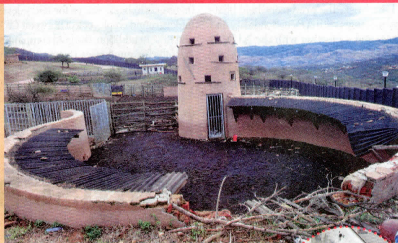
SHODDY: The crumbling chicken coop at President Zuma's house in Nkandla. PICTURE: HERBERT MPANGANE.
