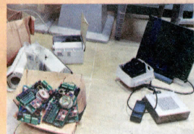
WHAT SECURITY?: Yet to be installed CCTV monitors at the police control room. PICTURE: GCIS.
