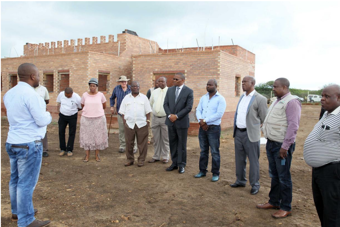
MEC Cyril Xaba together with Cllr Jeff Vilane Mthethwa and Cllr Bethuel Mthethwa at an Abattoir that is still under construction at Bhambanana, Jozini
